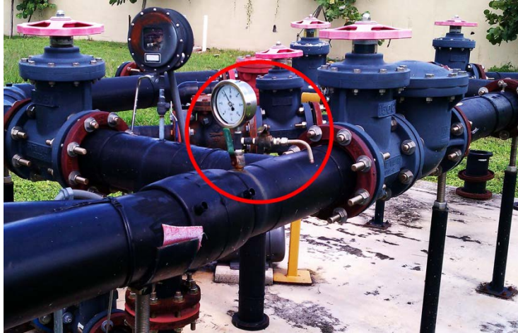
Figure 4: S.E. Step-up Station Sampling Port
