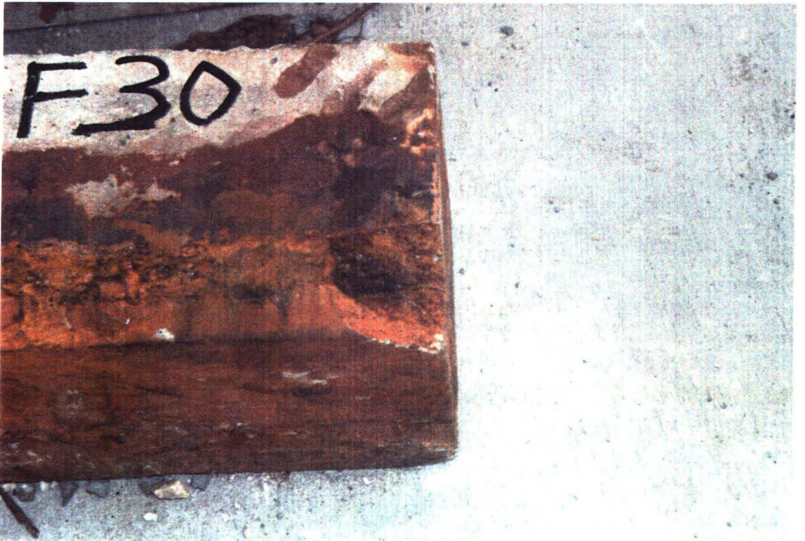
Fig. 5.2 Photographs of corroded beam specimens.
