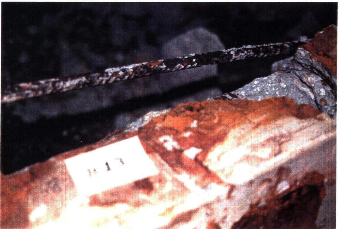
Fig. 5.3 Photographs of corrosion damage - Visible external crack and rebar corrosion.
