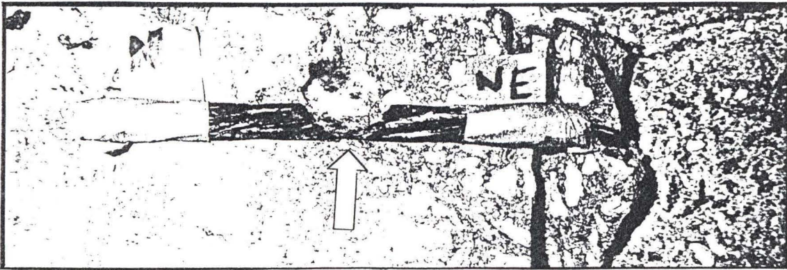
Figure 4-3: Cup shape corrosion at the NE pond for beam E6.
